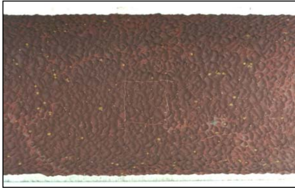
Figure 12 – The inner diameter of a steel tube that underwent erosion corrosion from exposure to contaminated water under turbulent flowing conditions shows a wavy morphology with evidence of oxidation. (0.6X)
